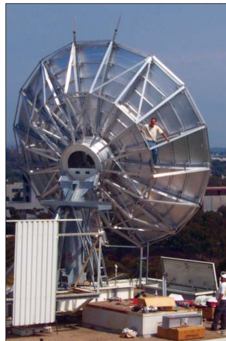
Fig. 1. One of the 7.2-meter HiSeasNet hub antennas being installed atop the San Diego Supercomputer Center (SDSC) building on the campus of the University of California, San Diego in La Jolla, Calif. The SDSC is the major regional node for the Internet.
